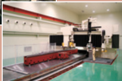
Temperature-controlled factory (Ultra-precision column-type surface grinding machine)
